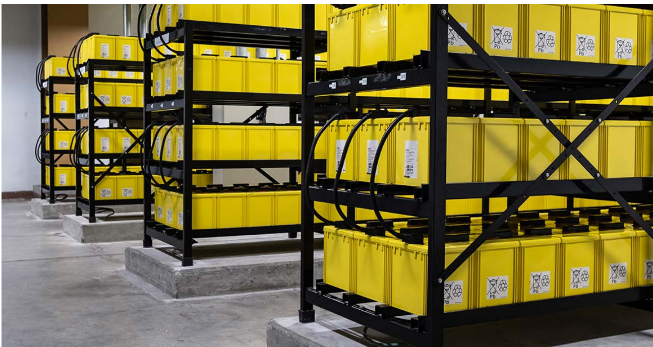
Figure 2: EnerSys® battery stacks deployed within a data center
